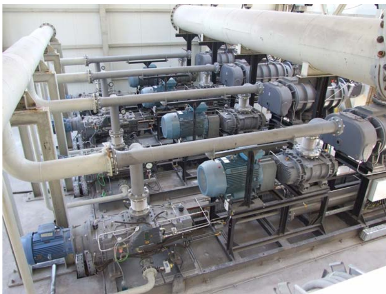
Figure 1 Typical modular dry pump installation for a 90 tonne VD process
